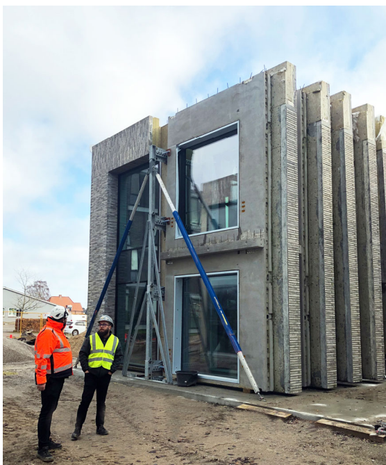
Caption: Safe intermediate storage for precast wall panels in the precast plant and on the construction site. © ROBUSTA-GAUKEL
